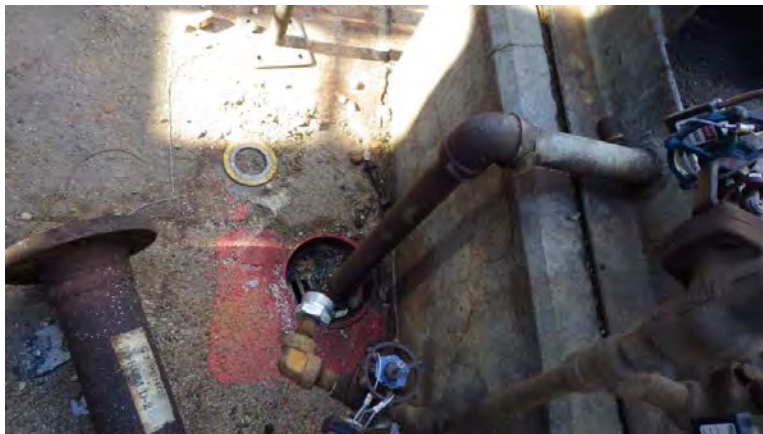
FIGURE 8. Typical pump drain to OWS (Source: CSB).
