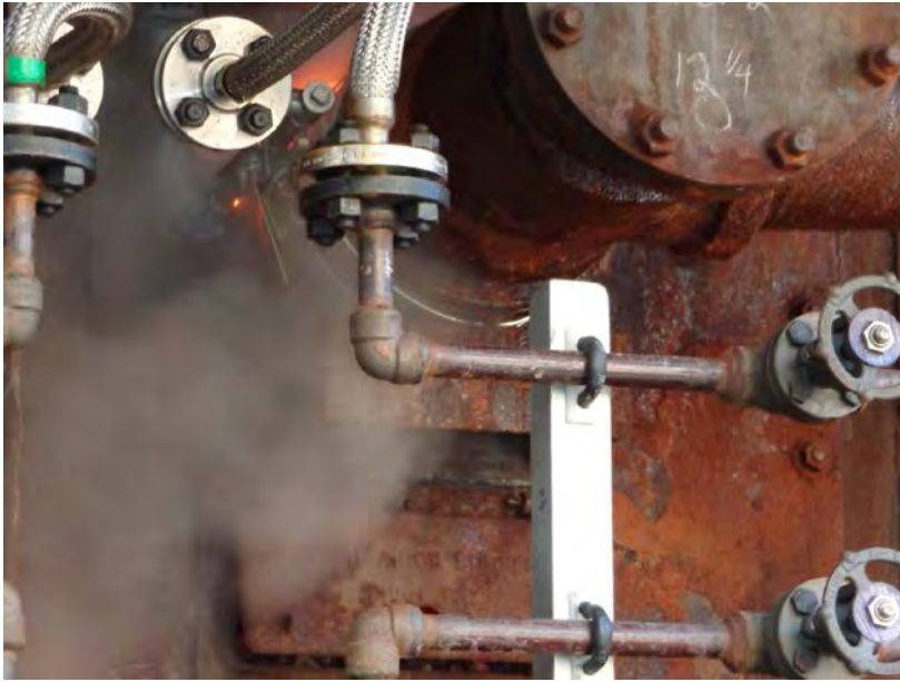
FIGURE 7. Burner on furnace (Source: CSB).
